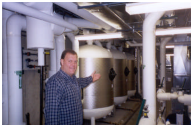
Larry Farley showing geothermal heat pump system.
