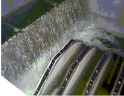
Cloth-media filter system used at CLSD for tertiary treatment.
