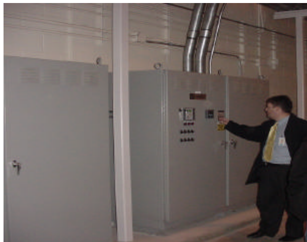
Bruce Jacobs points out features of energy monitoring equipment.
