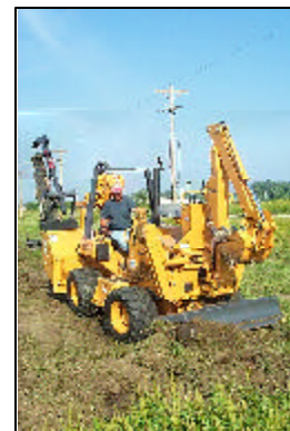
With the aid of equipment loaned by associate member Midwest Underground Supply, IAMU's Richard Nowels levels ground for IAMU's new training field storage building.
