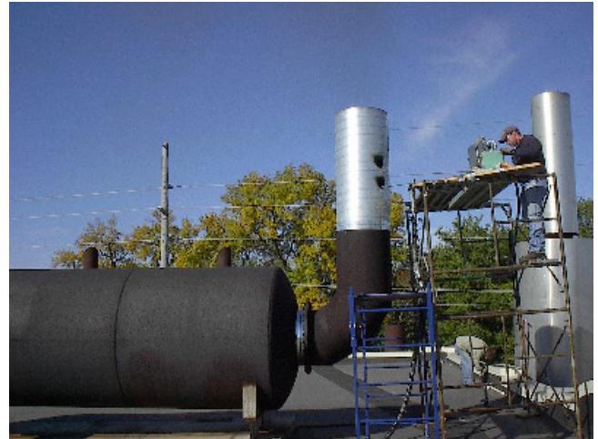
Figure 1 An example of the sampling probe setup in the stack on the roof top of a power plant
