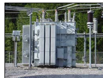
Electrical substations are just one example of infrastructure that is often rented by utilities, sometimes at a significant cost.
