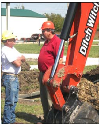
A special thanks to associate member Ditch Witch (representative Mike Wiedner is shown above, right) for their contributions of equipment and expertise for the IAMU Underground Electric Workshop.
