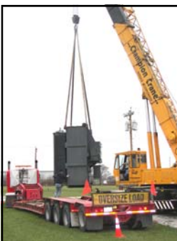
The Milford transformer arrives at IAMU and is unloaded on the Safety & Training Field.
