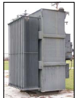
The transformer will be the cornerstone of a soon-to-be-constructed electric training substation.
