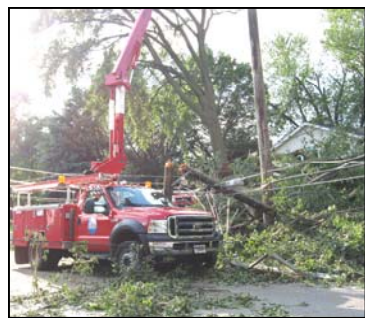
A challenging time for Cedar Falls Utilities. Power restoration was the order of the day following a storm packing 100+ mph winds July 10. The above photos show the type of damage seen in a wide area. Several IAMU member utilities assisted through IAMU's Mutual Aid Program (see the July 14 IAMU Informer).
