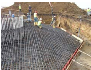
The foundations for WLP's Cannon I and Cannon II wind turbines were built last fall. The turbines blades and towers are set to arrive this week.
