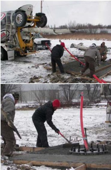
The foundation and base for IAMU's new wind turbine have been installed on the association's Safety & Training Field. The vertical axis wind turbine is scheduled to be in place this month.
